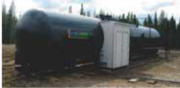
Vapor Tight Tanks
