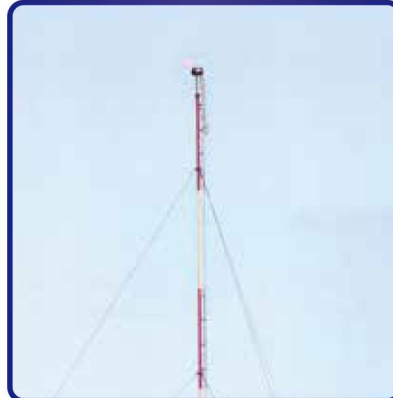
In service for months and there is no flame lick on flare tip or pilot. (increased dependability and service life)
