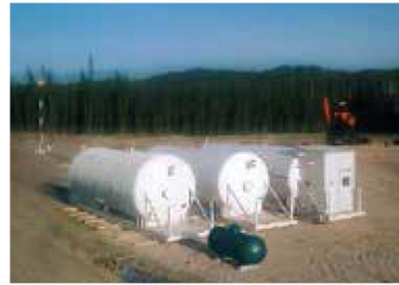
Gas Tight Production Packages
